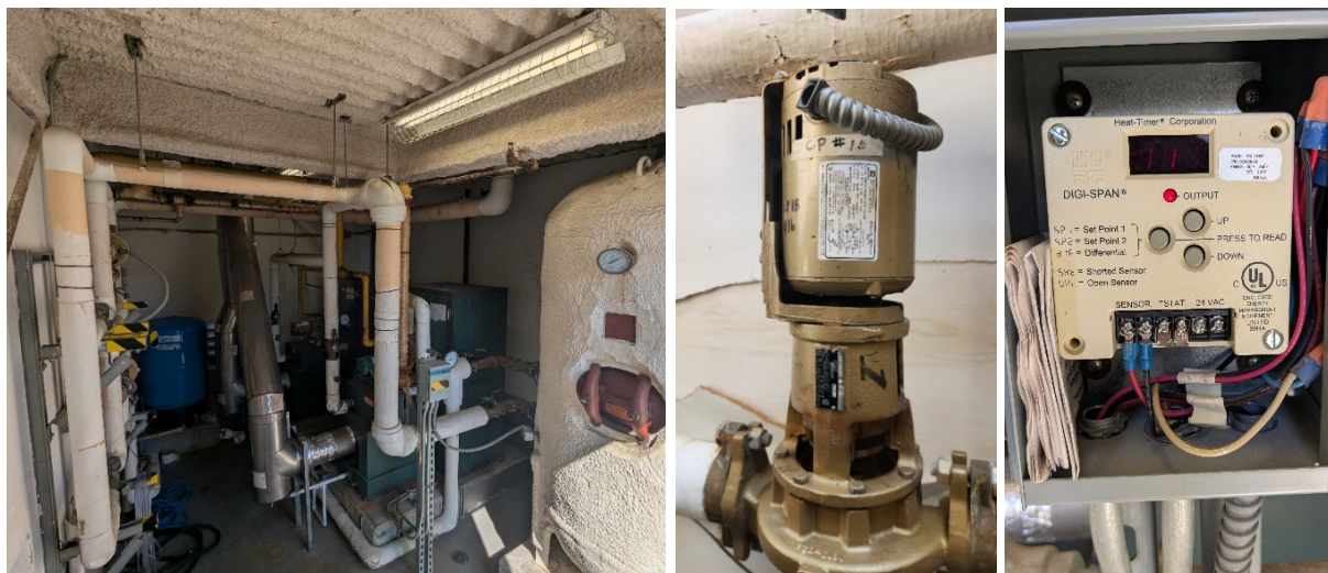
Figure 3: Site 1 DHW system mechanical room, recirculation pump, and controller.
