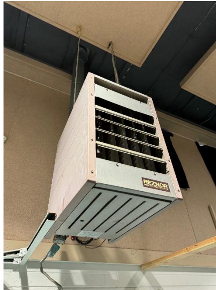
Figure C-27: Theatre Unit Heaters
