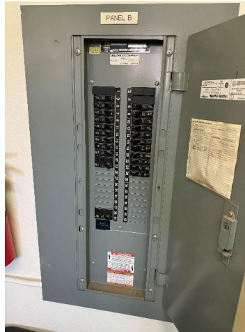
Figure C-25: "Panel B" Panelboard
