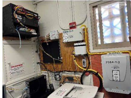
Figure C-30: Wireless Fiber Signal Box
