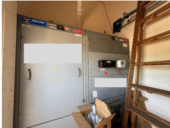
Figure C-15: Electric Meter and Switchboard
