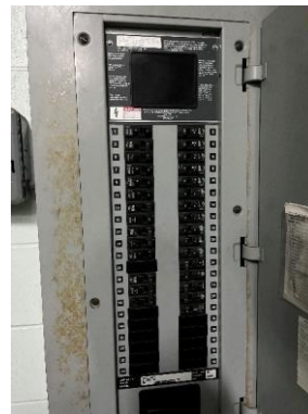
Figure C-33: Panelboard Serving Various Equipment
