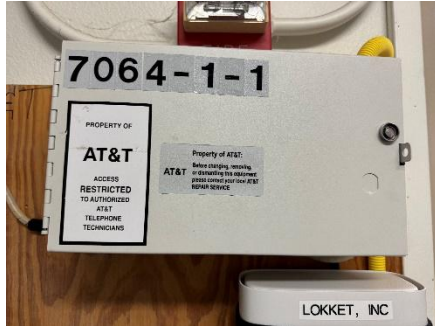
Figure C-29: Broadband Panel Box
