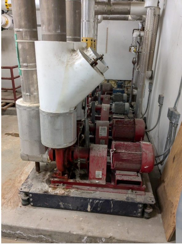
Figure 5: Existing hydronic pumps in the Dutton Hall mechanical room before the retrofit.
