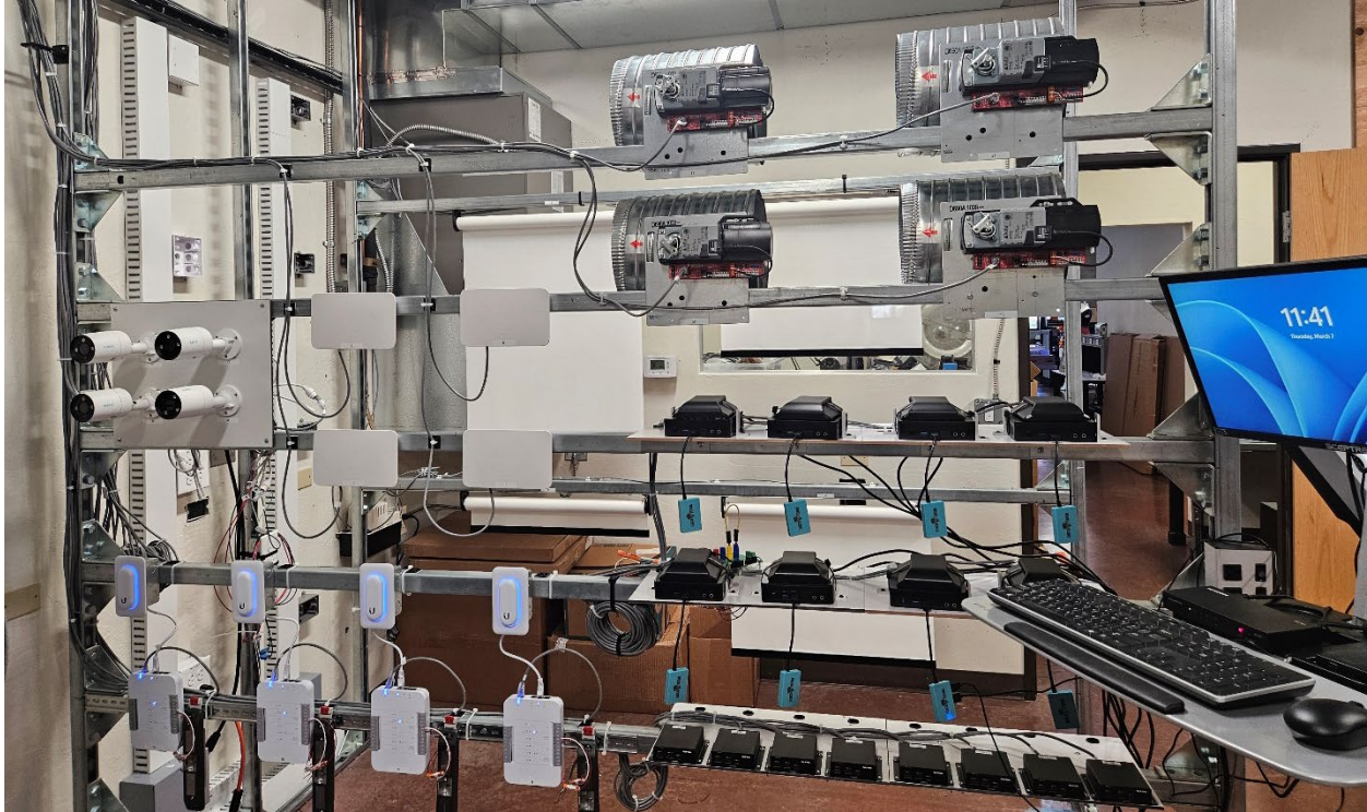
Figure 8: Rail mounted devices.
