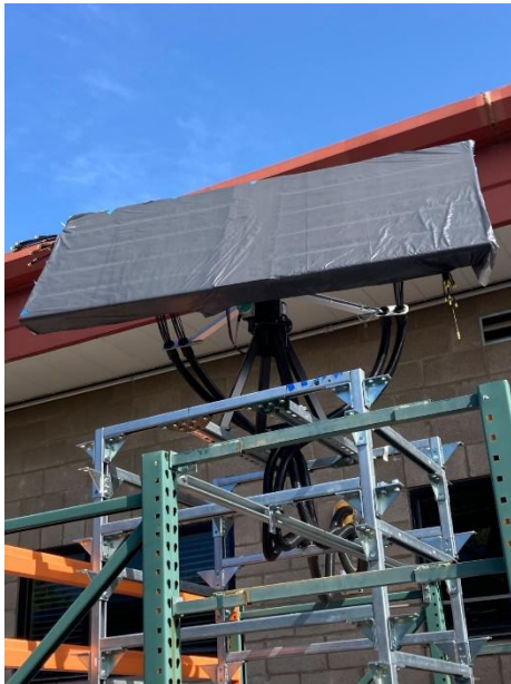
Figure 3: STF installation shown with optics covered.
