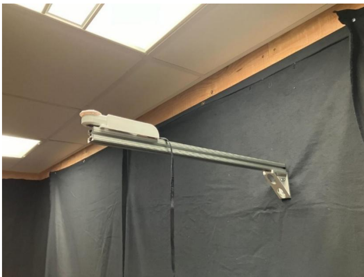
Figure 10: Control system illuminance sensor.
