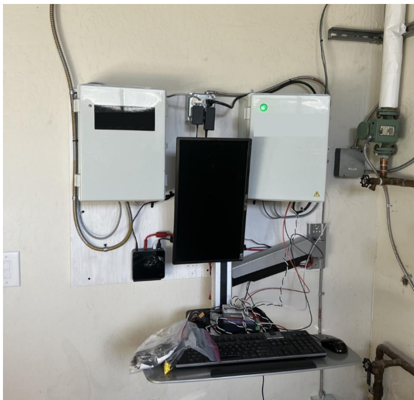
Figure 4: STF control board with power monitoring equipment.
