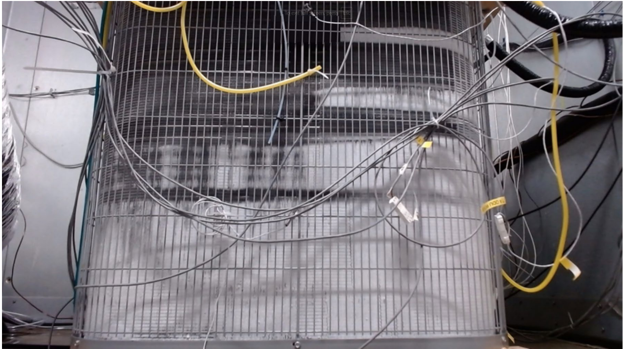
Figure 6. ODU midway through a defrost cycle.
