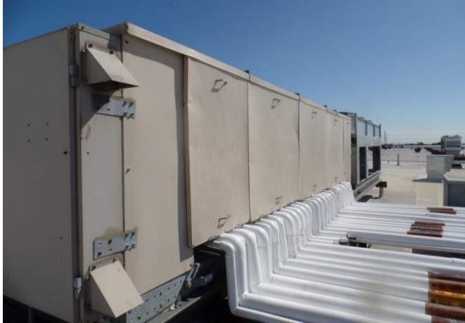
Figure 20: West Covina Rooftop Unit
