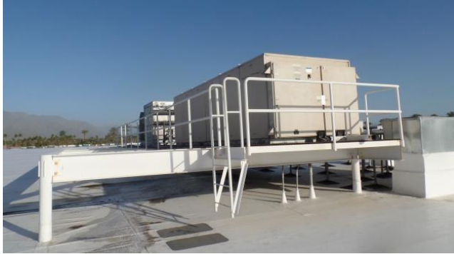
Figure 21: Cathedral City rooftop unit
