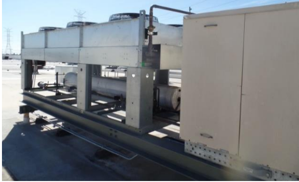
Figure 19: South Gate Rooftop Unit
