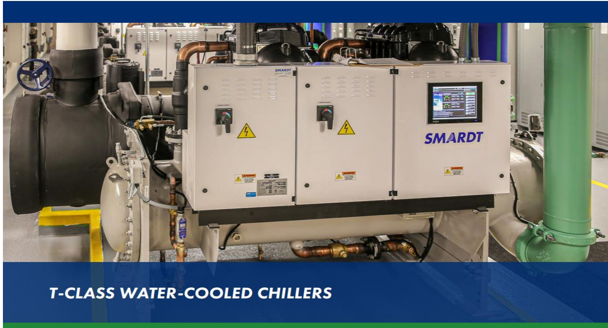
Figure 6: Smartd Oil free water cooled chillers
