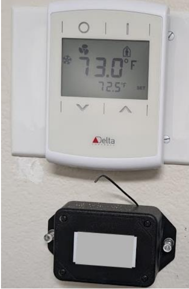
Figure 10: A thermostat and a temperature sensor installed in a zone.
