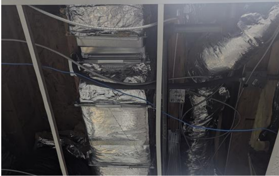
Figure 9: TESS modules installed in the supply duct in plenum.
