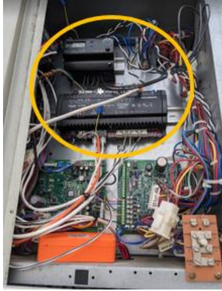
Figure 11: TESS a controller and an energy meter installed in AC4.
