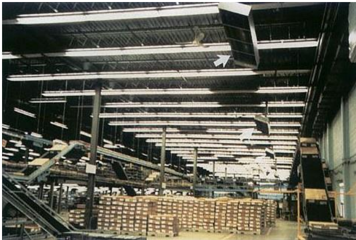
Figure 9: Low-intensity IR heaters in a clothing distribution center [26]
