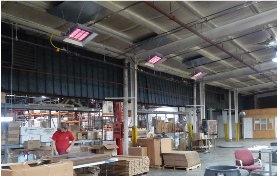
Figure 10: High-intensity IR heaters at a furniture plant [26]
