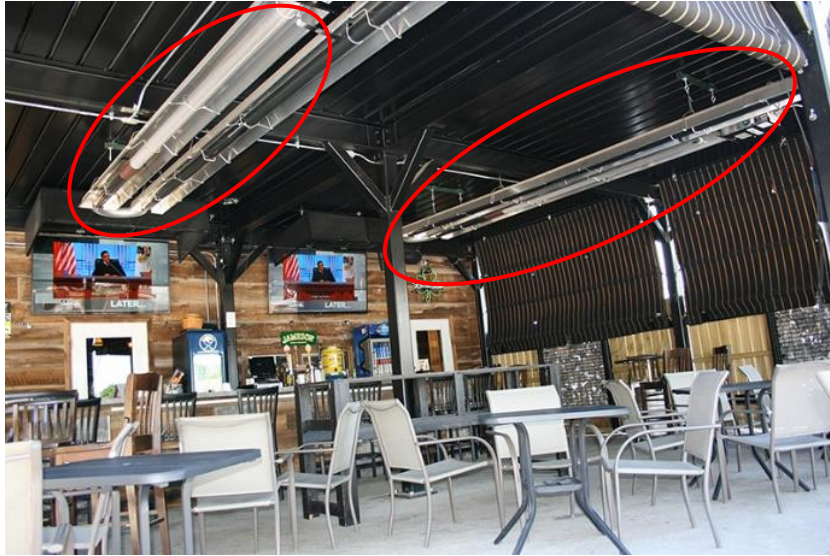
Figure 13: IR Heater for a restaurant in Illinois
