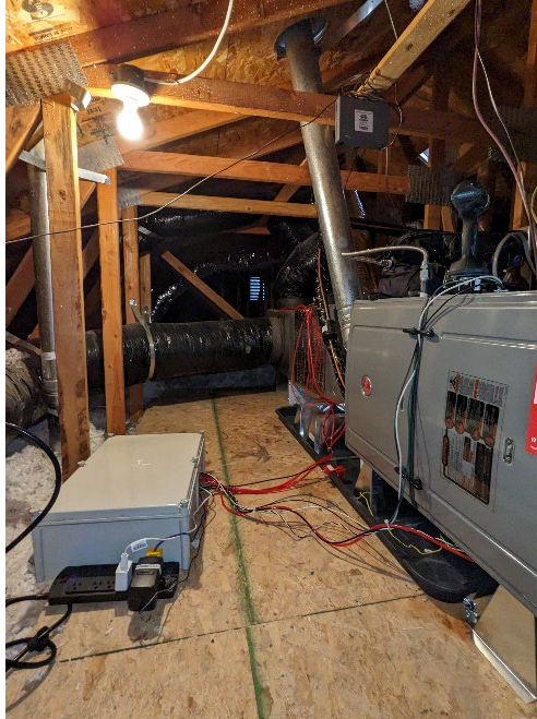
Figure 4. Data acquisition enclosure in attic of Site 2.
