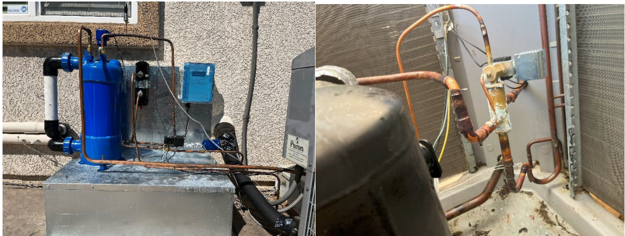
Figure 11. Photos of refrigerant components installed for the retrofit technology.
