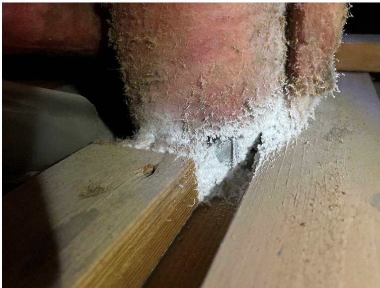
Figure 12. Sealant deposition on ductwork at register boot connection.
