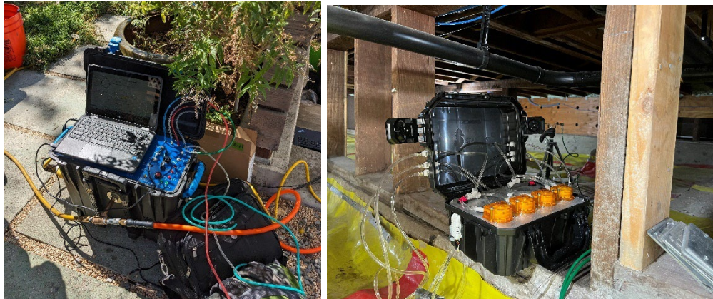
Figure 1. Aerosol sealing control unit (left) and remote injector unit (right).
