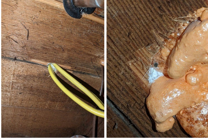
Figure 9. Seals formed at penetrations in the floorboard at Site 1
