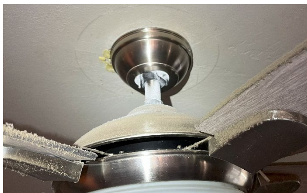
Figure 11. Buildup of sealant on ceiling fan.
