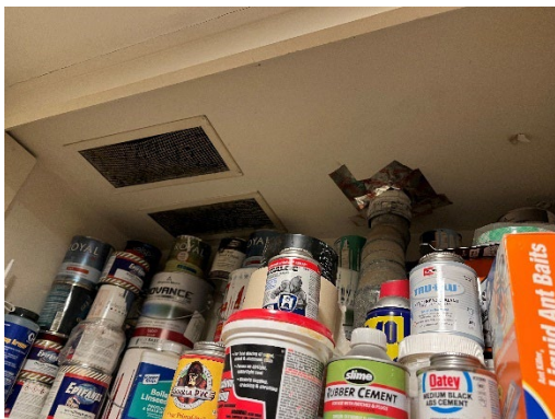
Figure 7. Makeup air grilles between the attic and water heater location in the home.
