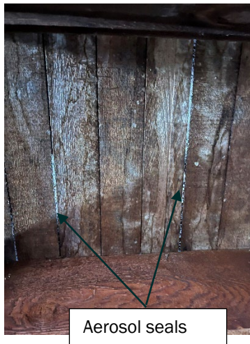
Figure 10. Example seals formed between floorboards at Site 2.
