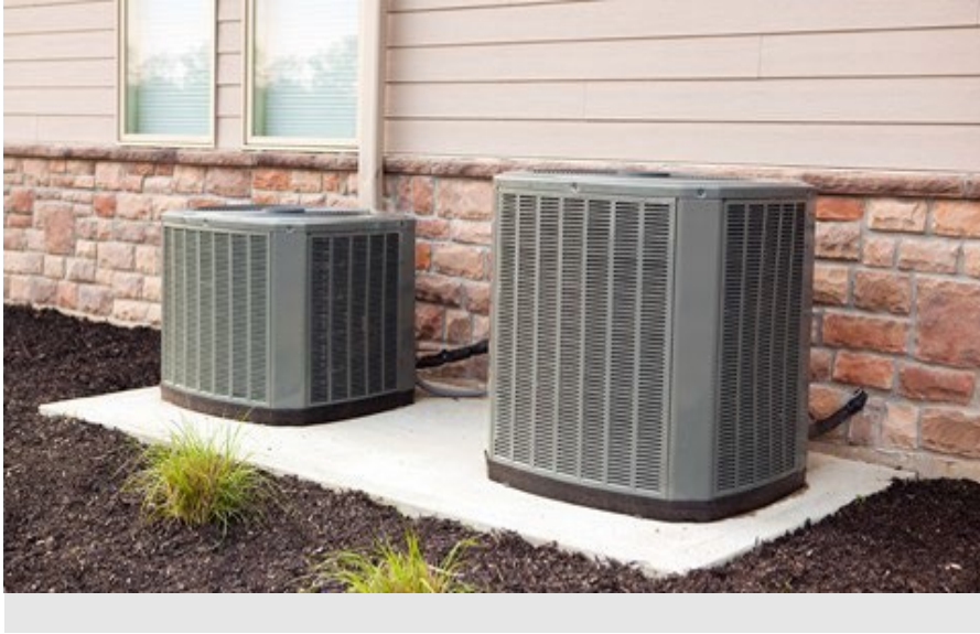
Figure 3: Image of CAC outside condenser units and refrigerant line sets penetrating masonry wall (courtesy of Efficiency Vermont).
