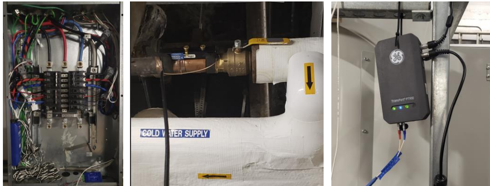
Figure 6: Swing tank power metering and city water ultrasonic pipe surface flow metering
