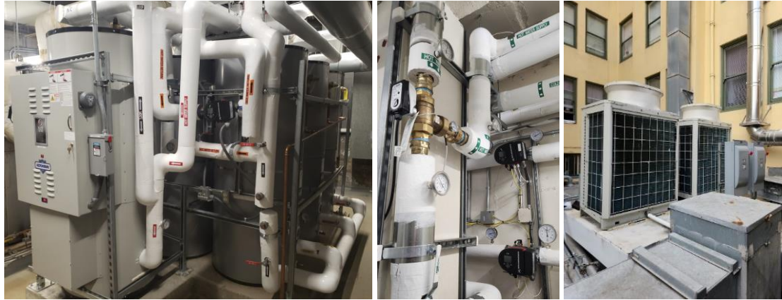
Figure 3: Swing tank and storage tank array, mixing valve, and rooftop HPWHs.
