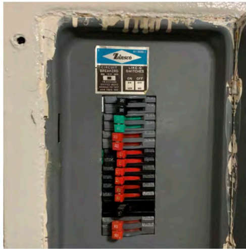
Electrical Panel label photo example
