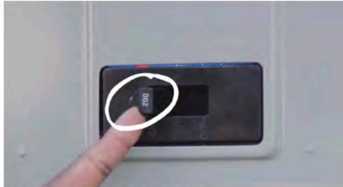
'Main circuit breaker' or 'main breaker'
