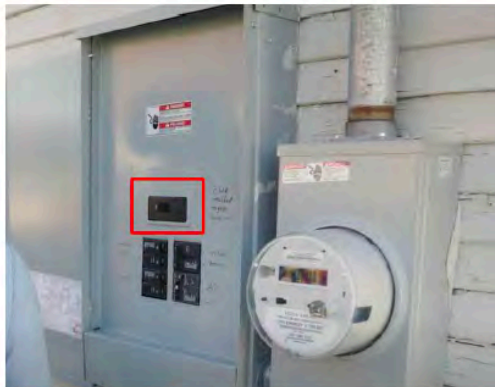
Main breaker next to electrical meter
