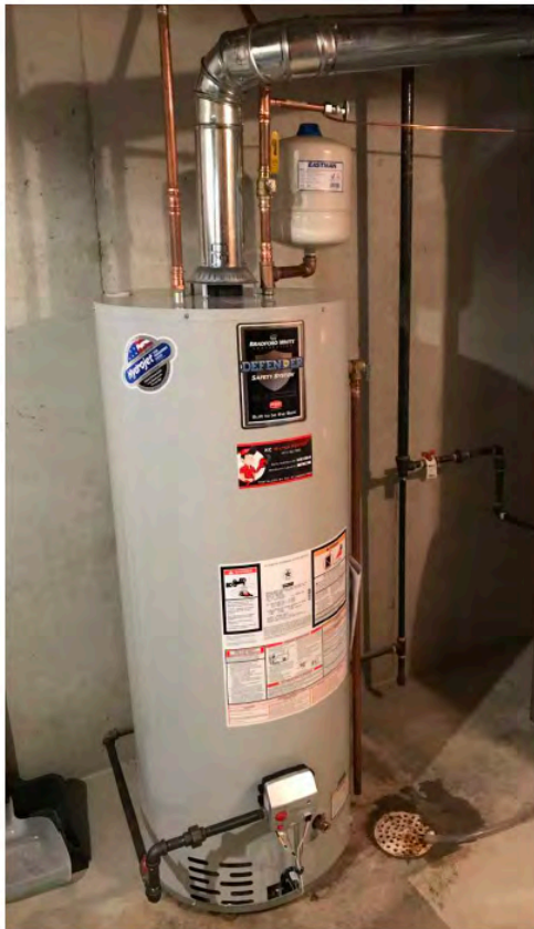
Storage Tank - Gas water heater
