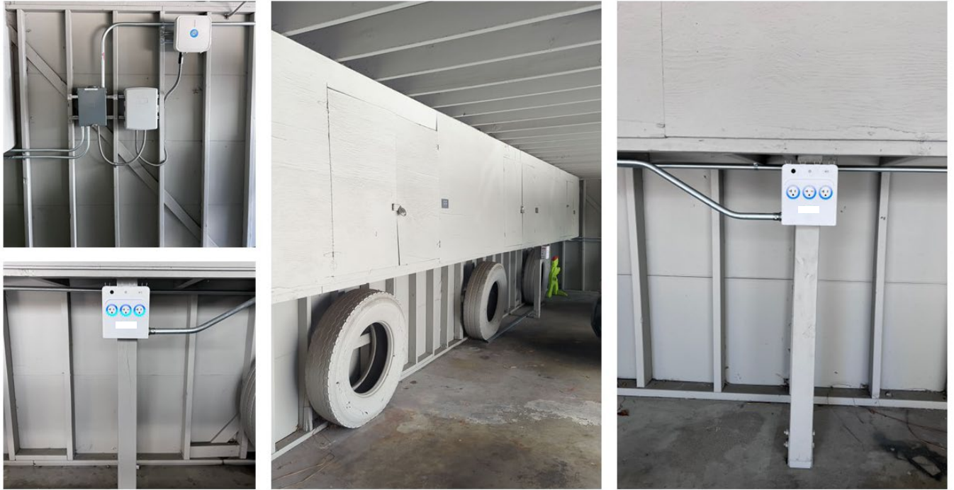
Figure 24: Installed chargers at Site 2 wired from the house panel, and the dedicated electrical panel which will power the full installation once the utility upgrades the service.
