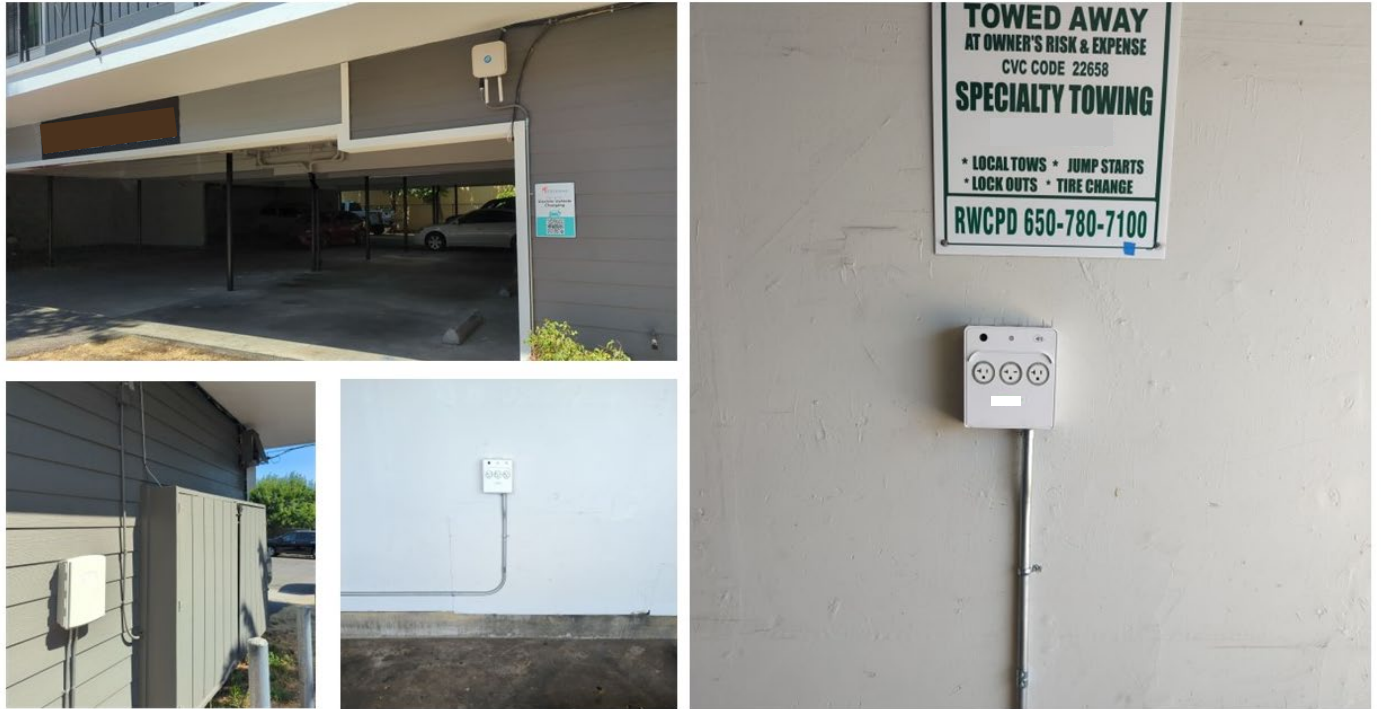
Figure 26: Installed chargers at Site 4 wired from the house panel and images of the LCU apparatus for the installed chargers.
