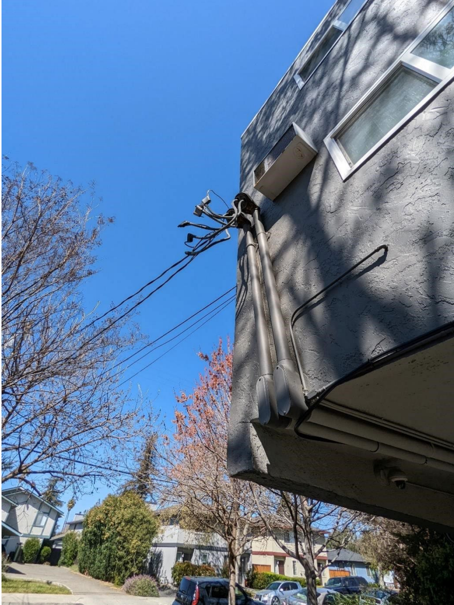
Figure 25: This is the aerial drop which the utility stated cannot handle any more electrical load at the building. The utility must upgrade it before the full installation can be finalized.
