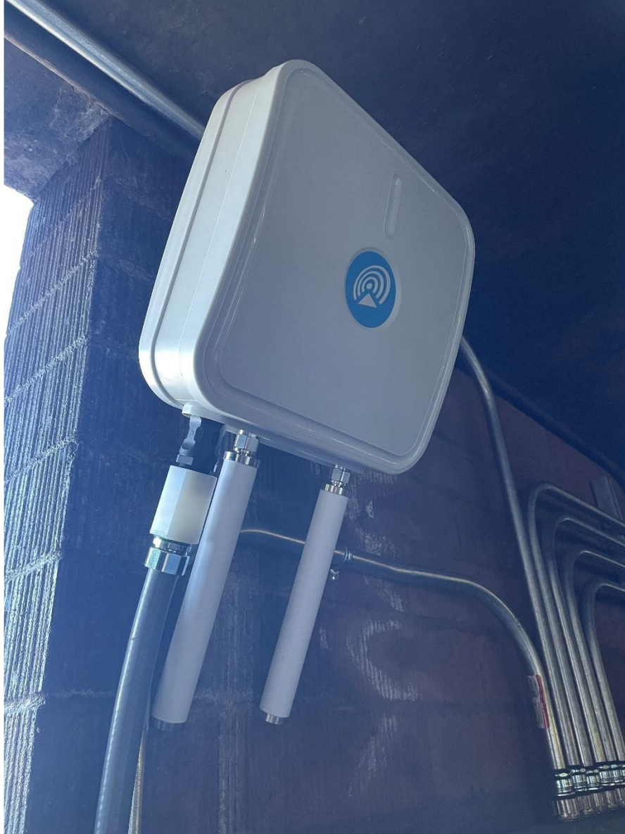
Figure 20: Local Control and Uplink (LCU) at Site 1
