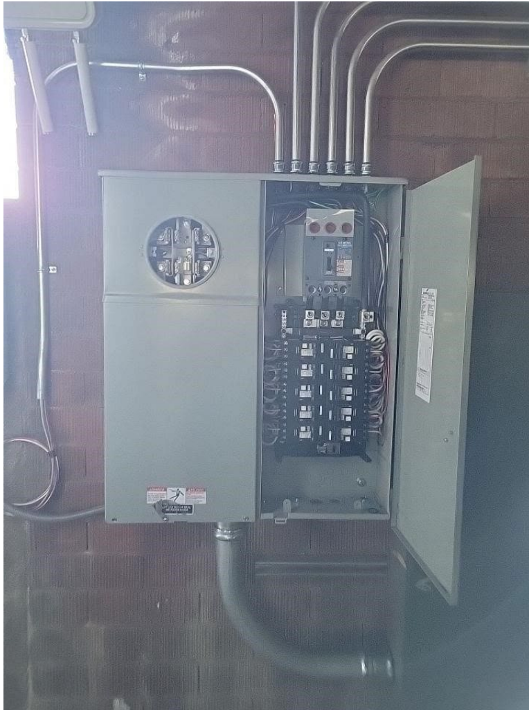
Figure 21: Evaluated Technology Provider Electrical Panel at Site 1
