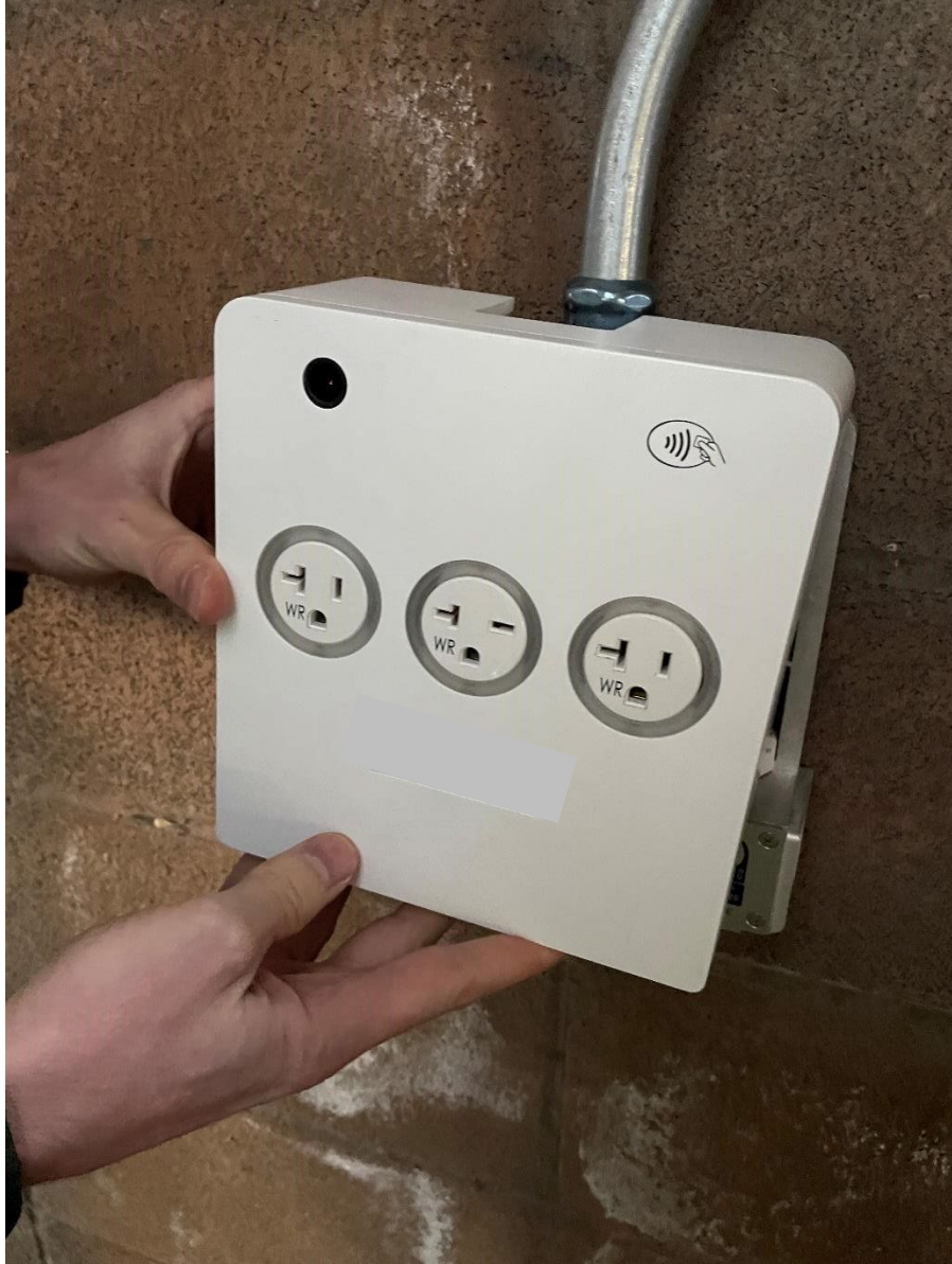
Figure 19: Charging Unit at Site 1
